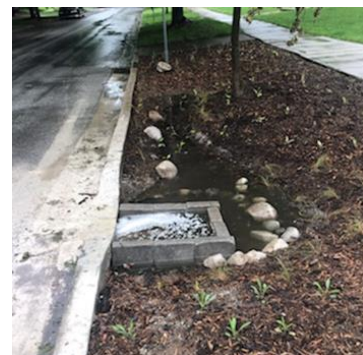
Fig. 3: A sediment trap in a rain garden filling with water, and depositing sediment into the trap that would have ultimately ended up in Plaster Creek.
