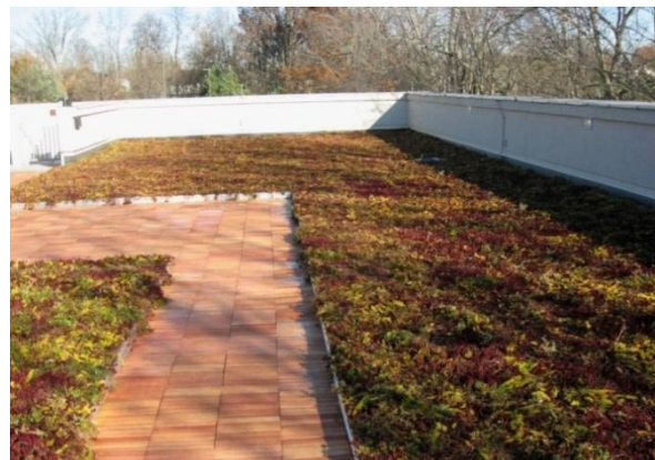
Figure 5-4. Green roof example.
