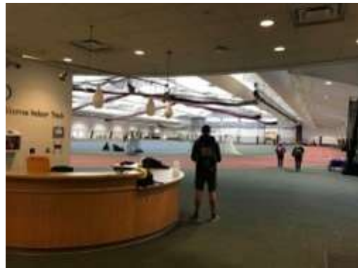
Figure D2. 2: Energy Efficient Case: LED Lights in TNT
