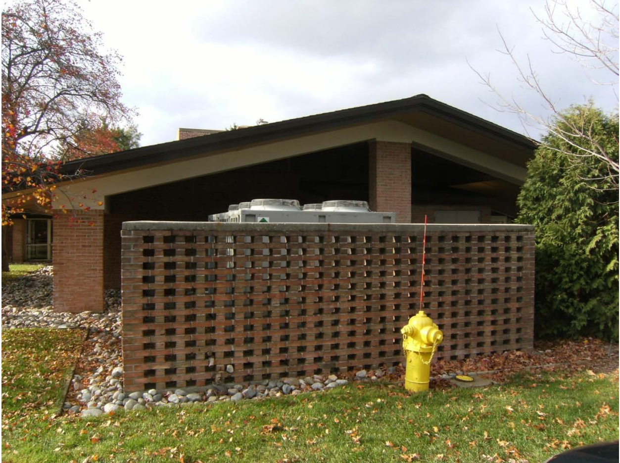
Figure 1: Picture of air cooled chillers at Calvin Seminary
